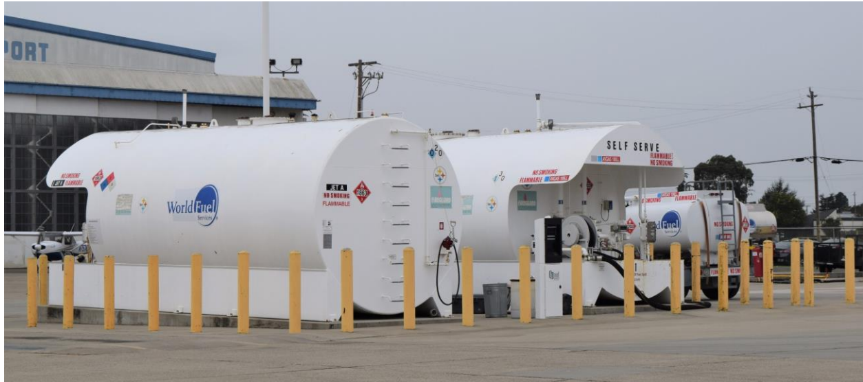
Figure 1.25 – World Fuel/Jet West Fuel Farm
