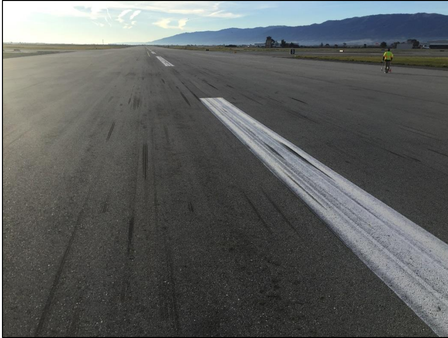
Runway 13-31, Section 10C – Weathering
