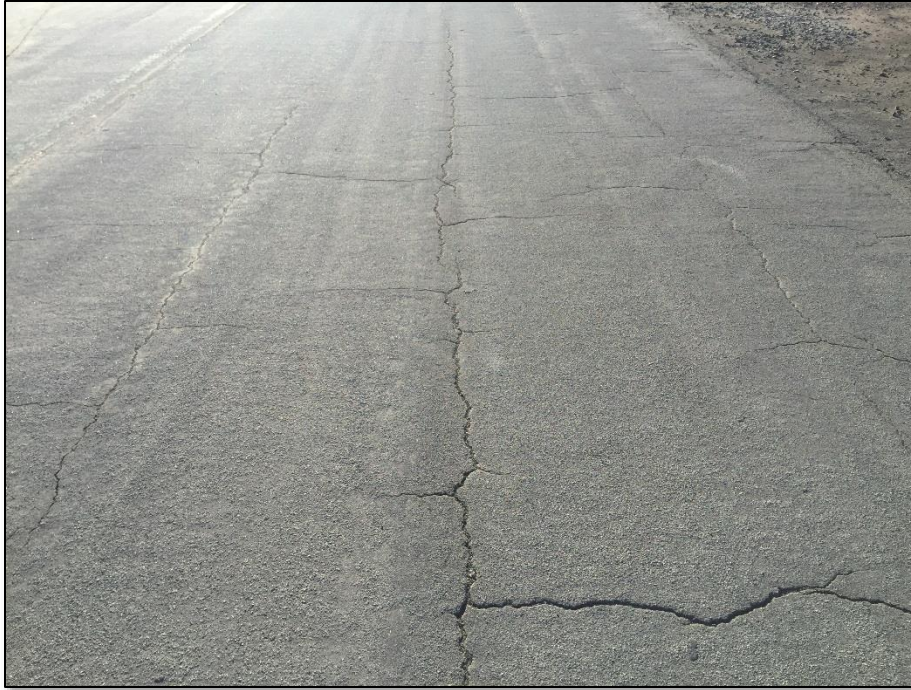
Taxiway G, Section 10 – Block Cracking
