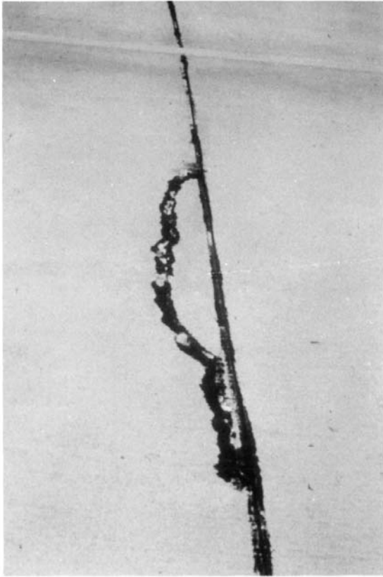
FIG. X2.62 Low-Severity Joint Spall
