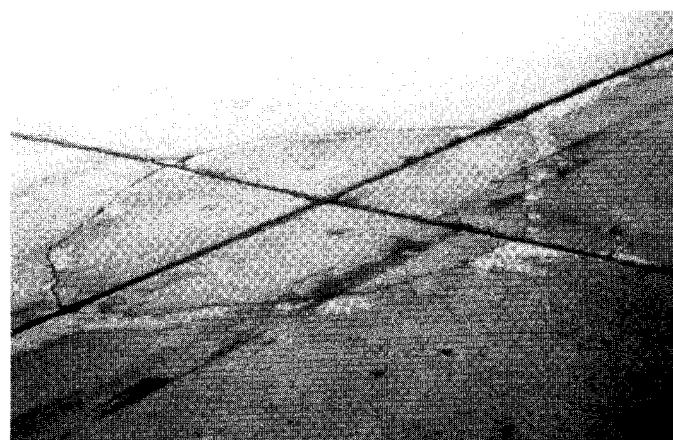
FIG. X2.4 Low-Severity Corner Break
