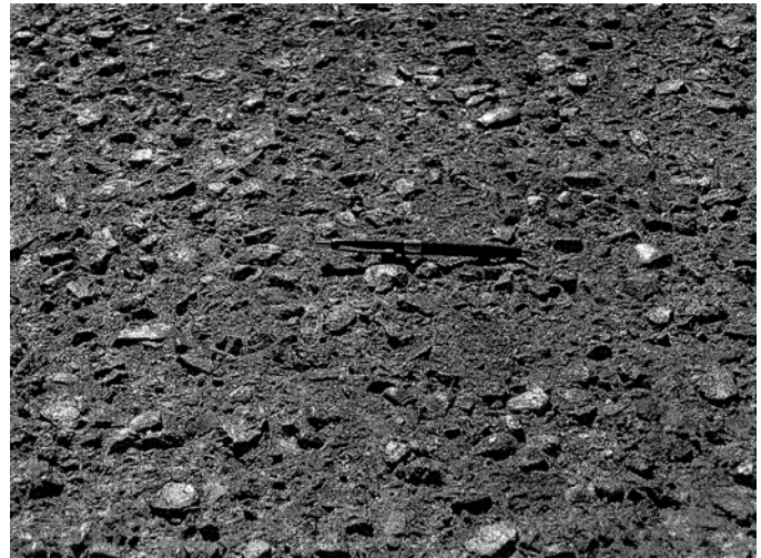
FIG. X1.81 High-Severity Weathering (Surface Wear)
