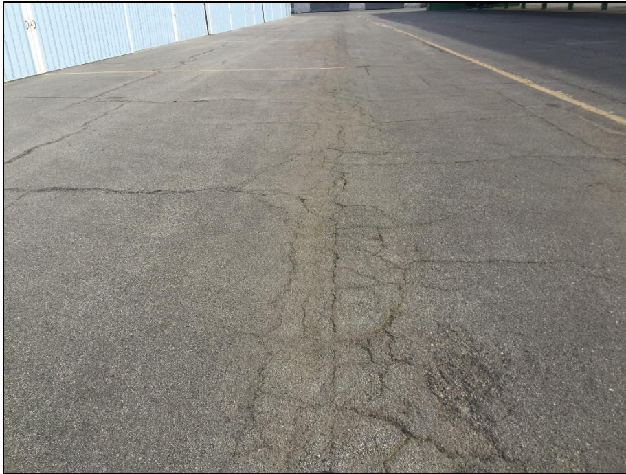
North Hangar Apron, Section 20 – Alligator Cracking
