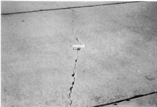
FIG. X2.14 Medium-Severity Transverse Crack
