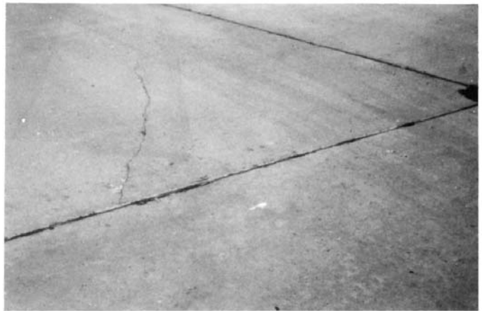
FIG. X2.11 Low-Severity Diagonal Crack
