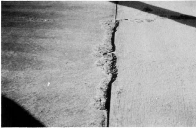
FIG. X2.67 High-Severity Joint Spall
