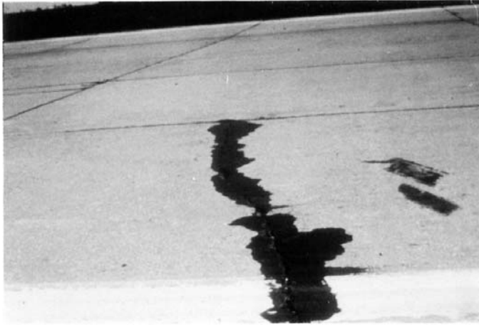
FIG. X2.13 Medium-Severity Transverse Crack
