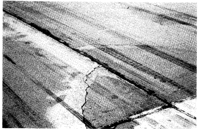
FIG. X2.7 Medium-Severity Corner Break
