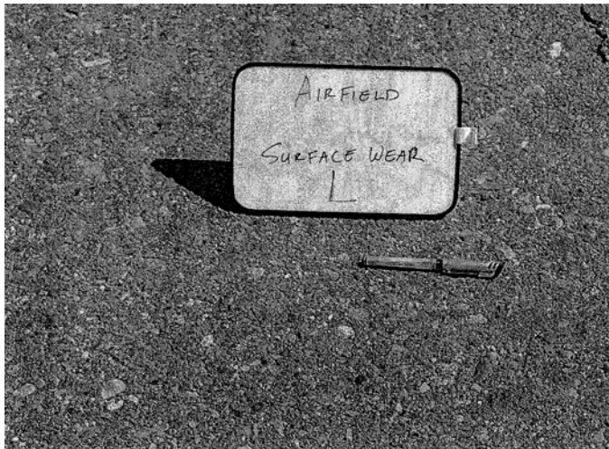
FIG. X1.79 Low-Severity Weathering (Surface Wear)
