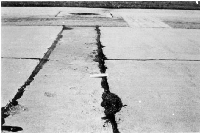
FIG. X2.36 Medium-Severity Utility Cut
