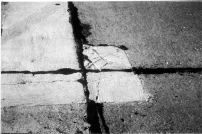
FIG. X2.31 Medium-Severity Small Patch
