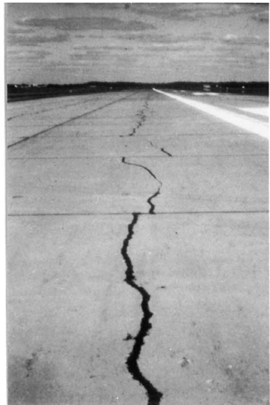
FIG. X2.12 Medium-Severity Longitudinal Crack
