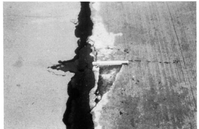
FIG. X2.65 Medium-Severity Joint Spall
