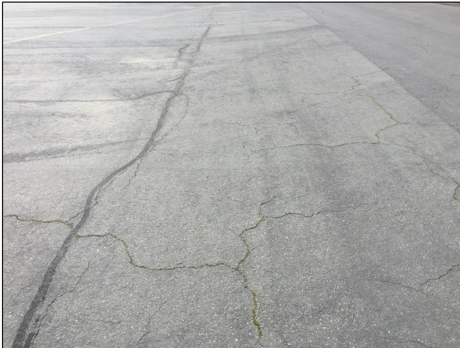
Tie Down Apron, Section 30 – Block Cracking
