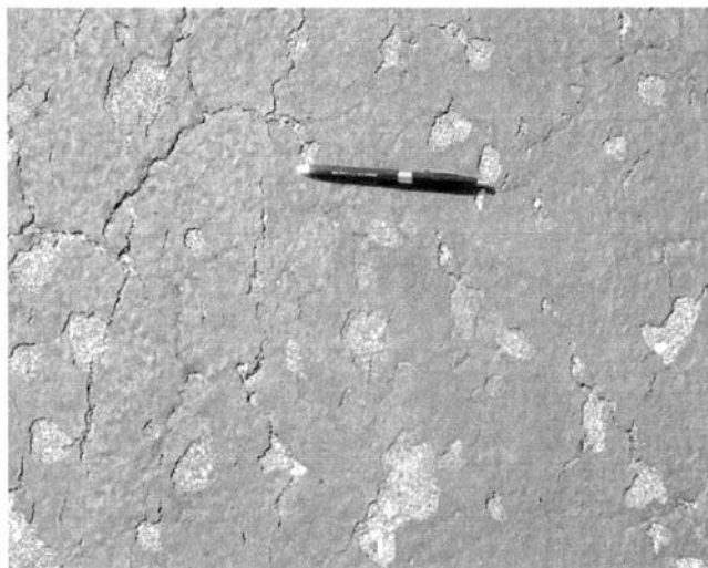
FIG. X1.60 High-Severity Raveling, Cold Tar
