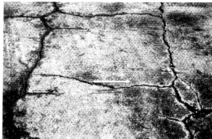
FIG. X1.16 Medium-Severity Block Cracking
