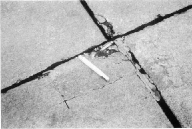
FIG. X2.30 Medium-Severity Small Patch
