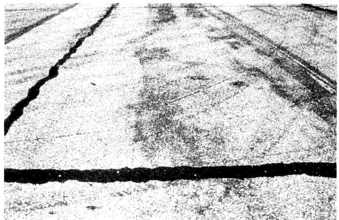
FIG. X1.31 Low-Severity Joint Reflection Cracking, Filled Crack
