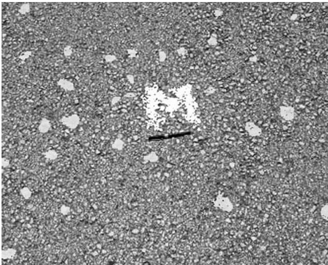
FIG. X1.56 Medium-Severity Raveling, Dense Mix
