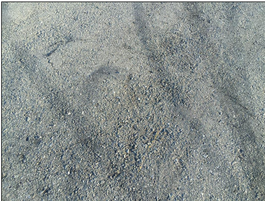
Taxiway D, Section 30 – Raveling
