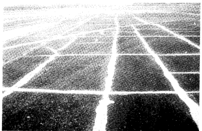
FIG. X1.13 Low-Severity Block Cracking, Filled Cracks
