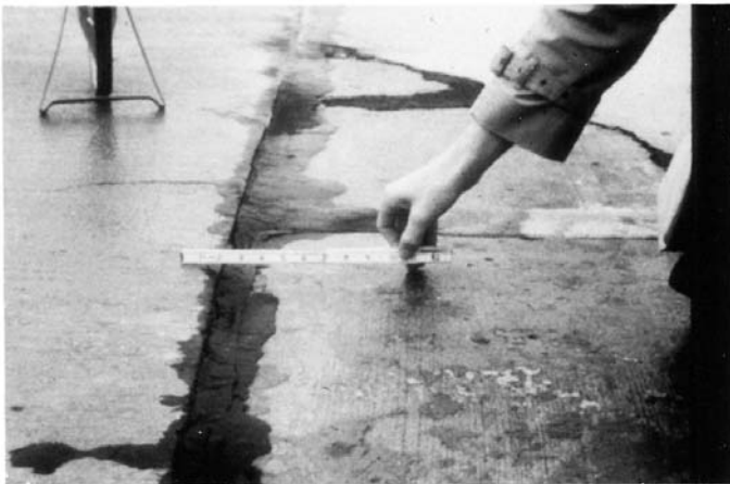
FIG. X2.50 Medium-Severity Settlement on Apron ( >1/2 in. (13 mm))
