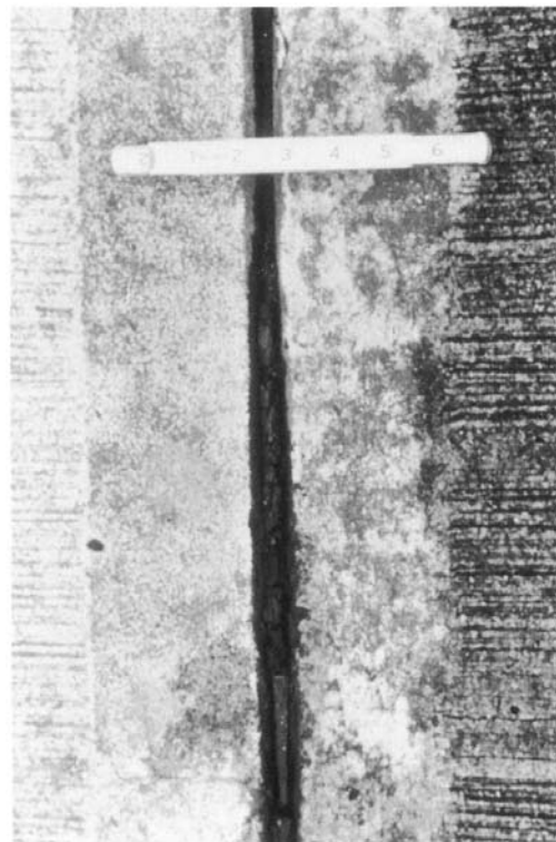
FIG. X2.25 Medium-Severity Joint Seal Damage (Note that Sealant has Lost Bond and is Highly Oxidized)
