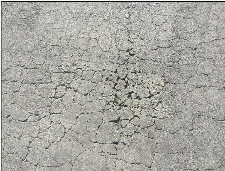
North Hangar Apron, Section 10 – Alligator Cracking
