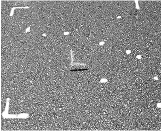
FIG. X1.55 Low-Severity Raveling, Dense Mix
