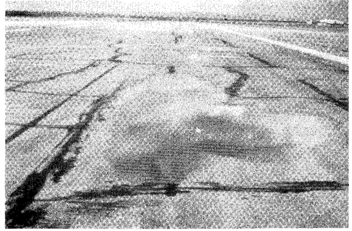
FIG. X1.27 High-Severity Depression (2 in. (50 mm))
