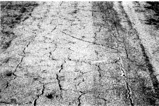
FIG. X1.20 High-Severity Block Cracking
