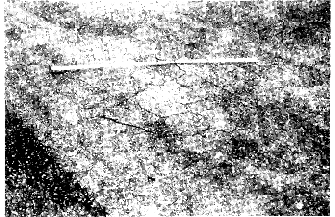
FIG. X1.7 Medium-Severity Alligator Cracking, Approaching High Severity (Example 1)
