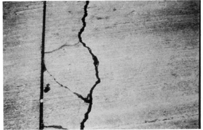
FIG. X2.64 Medium-Severity Joint Spall
