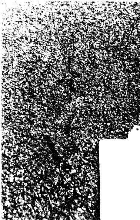
FIG. X1.44 Medium-Severity Crack in Porous Friction Course
