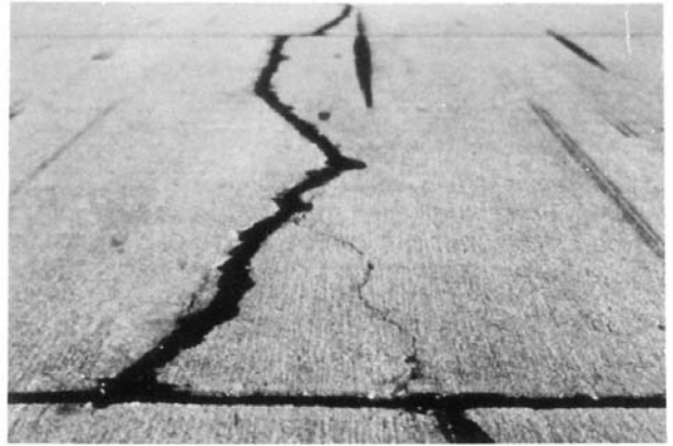
FIG. X2.16 High-Severity Longitudinal Cracks
