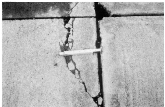
FIG. X2.71 Medium-Severity Corner Spall
