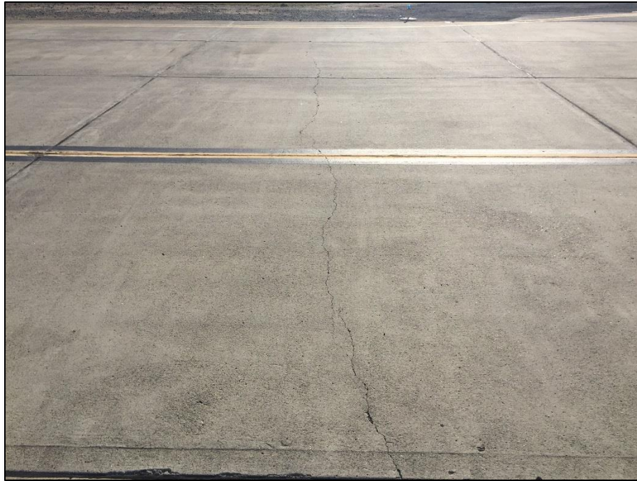
Taxiway F, Section 10 – Transverse Cracking
