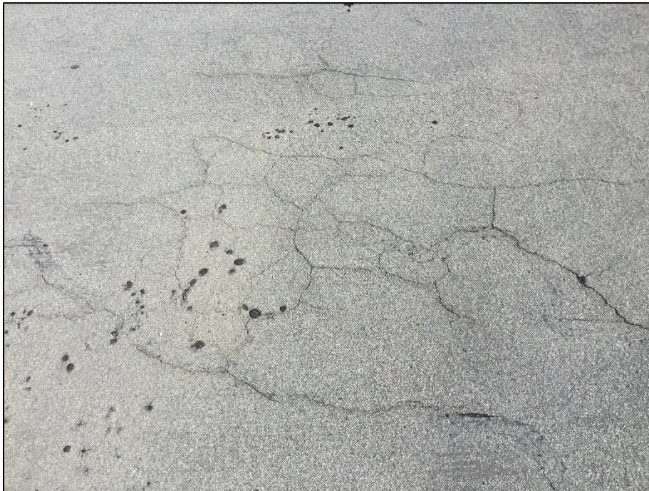
Taxiway J, Section 10 – Alligator Cracking
