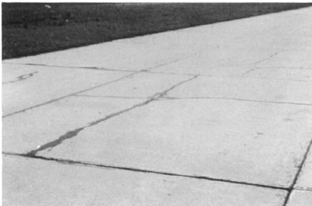
FIG. X2.56 Medium-Severity Intersecting Cracks
