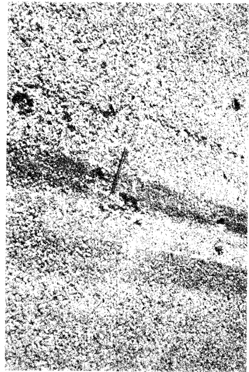
FIG. X1.65 High-Severity Raveling on a Porous Friction Course Surface
