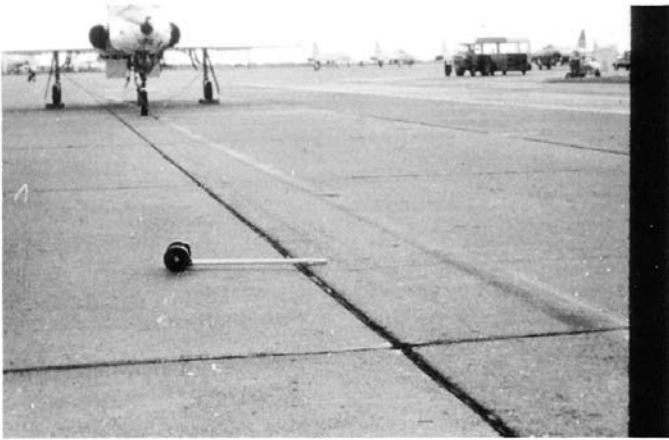
FIG. X2.49 Low-Severity Settlement on Apron
