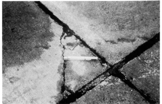
FIG. X2.70 Medium-Severity Corner Spall
