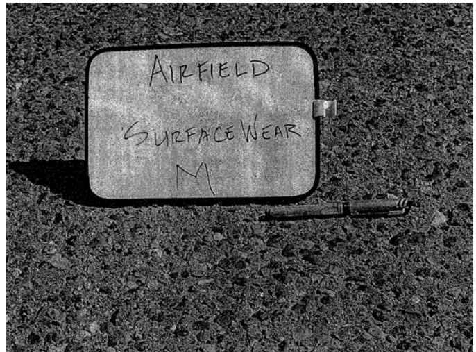
FIG. X1.80 Medium-Severity Weathering (Surface Wear)
