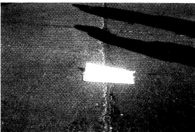
FIG. X1.34 Medium-Severity Joint Reflection Cracking
