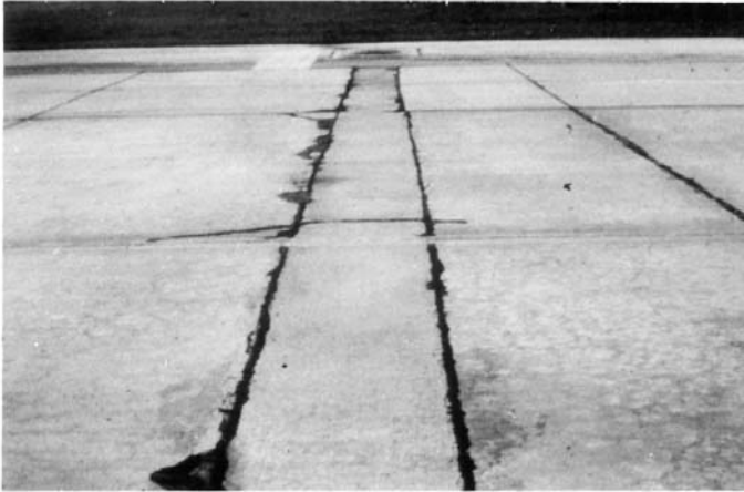
FIG. X2.35 Low-Severity Utility Cut
