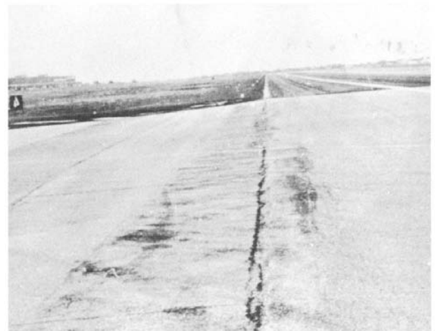
FIG. X1.71 Shove of Low Severity on the Outside and Medium Severity in the Middle
