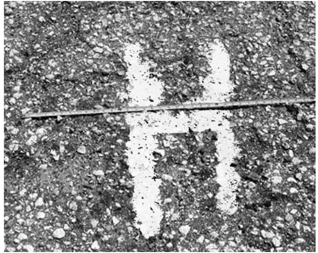
FIG. X1.57 High-Severity Raveling, Dense Mix
