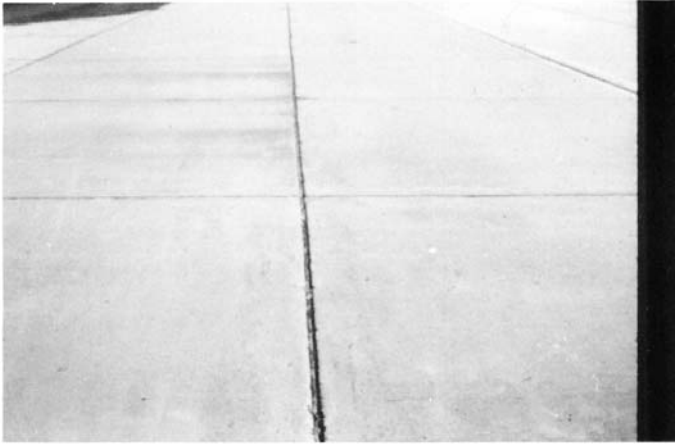
FIG. X2.40 Pumping (Note Stains on Pavement)
