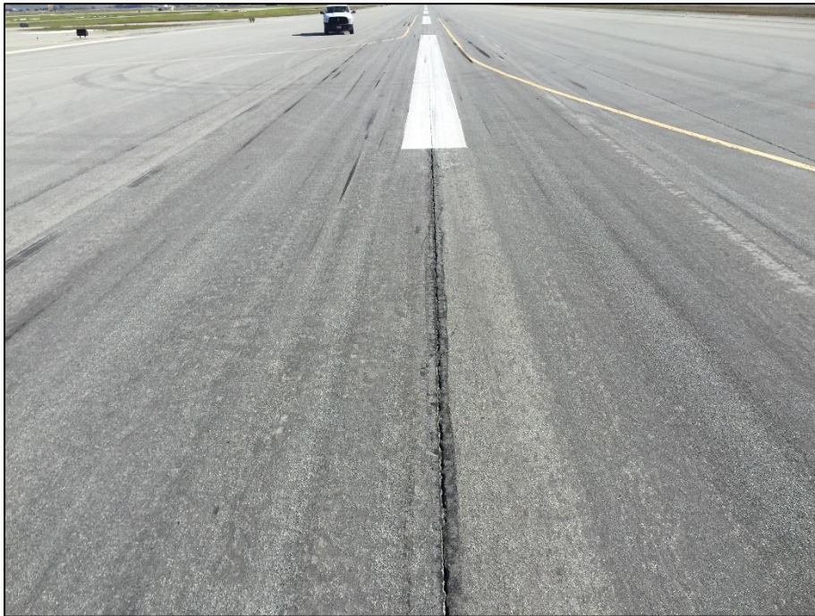
Runway 08-26, Section 10C – Longitudinal and Transverse Cracking and Raveling
