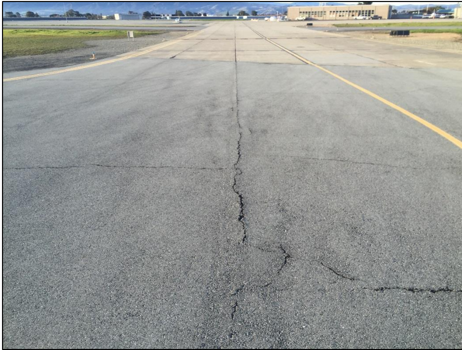
Taxiway F, Section 20 – Joint Reflection Cracking
