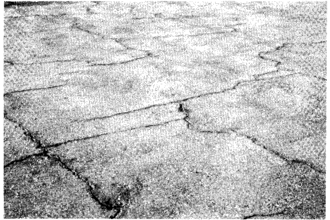
FIG. X1.17 Medium-Severity Block Cracking
