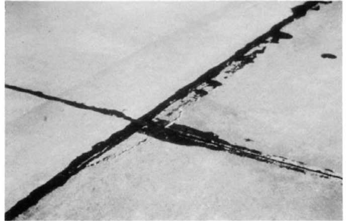
FIG. X2.69 Low-Severity Corner Spall
