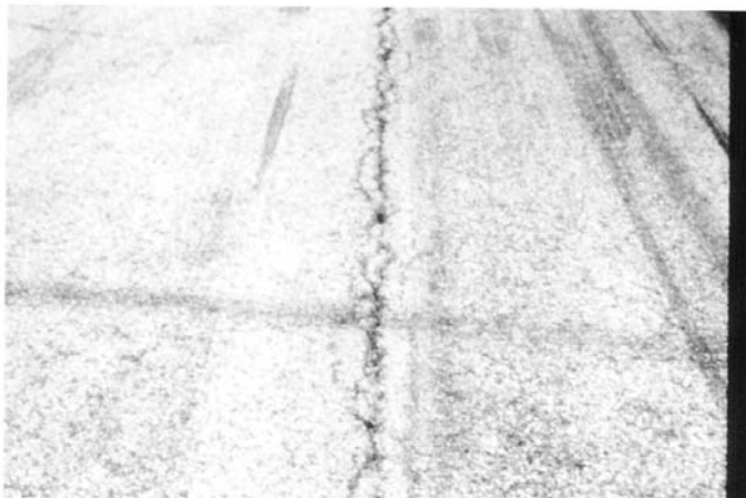
FIG. X1.39 Medium-Severity Longitudinal Construction Joint Crack
