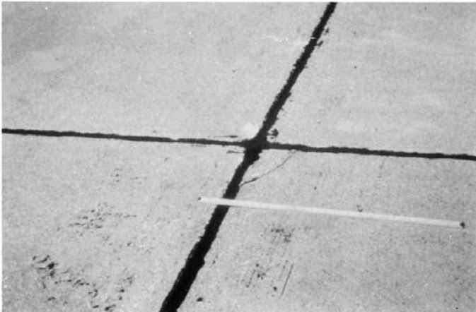
FIG. X2.68 Low-Severity Corner Spall
